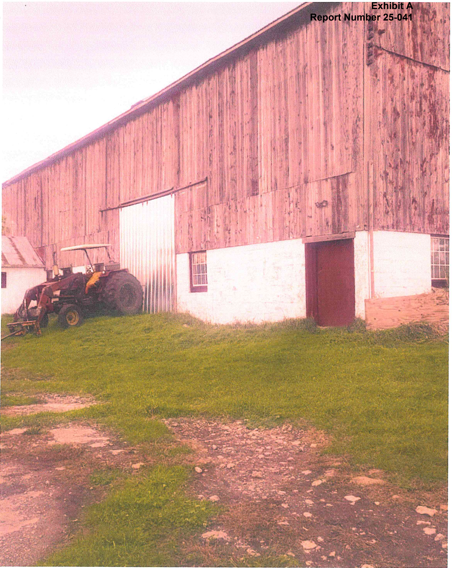
We replaced broken windows, new wood where it was missing, new doors, nailed down loose roof tin.
