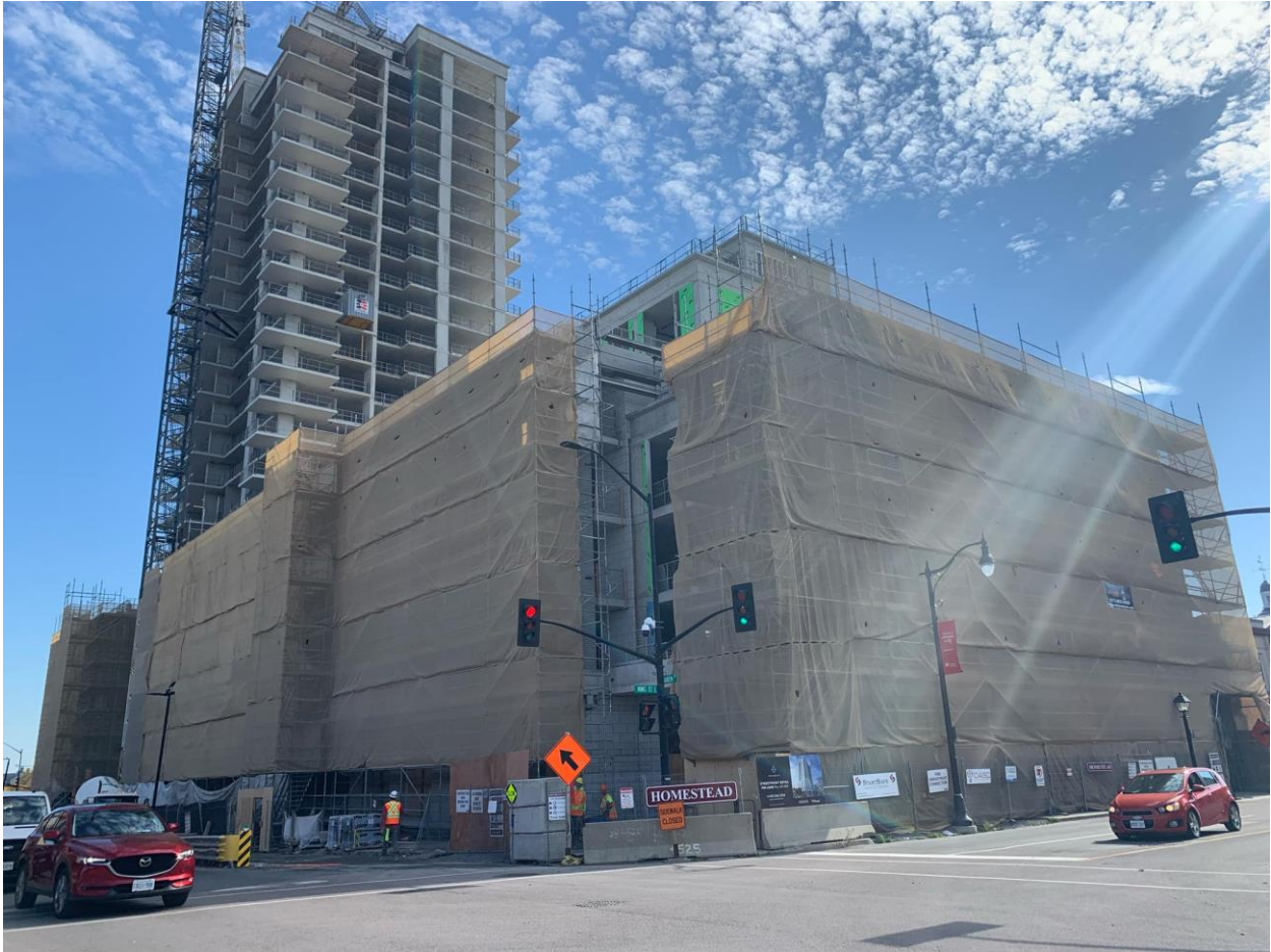
Figure 6: View of 18 Queen Street and 282 Ontario Street, currently under construction, located southeast of the subject property on Queen Street (October 22, 2024).
