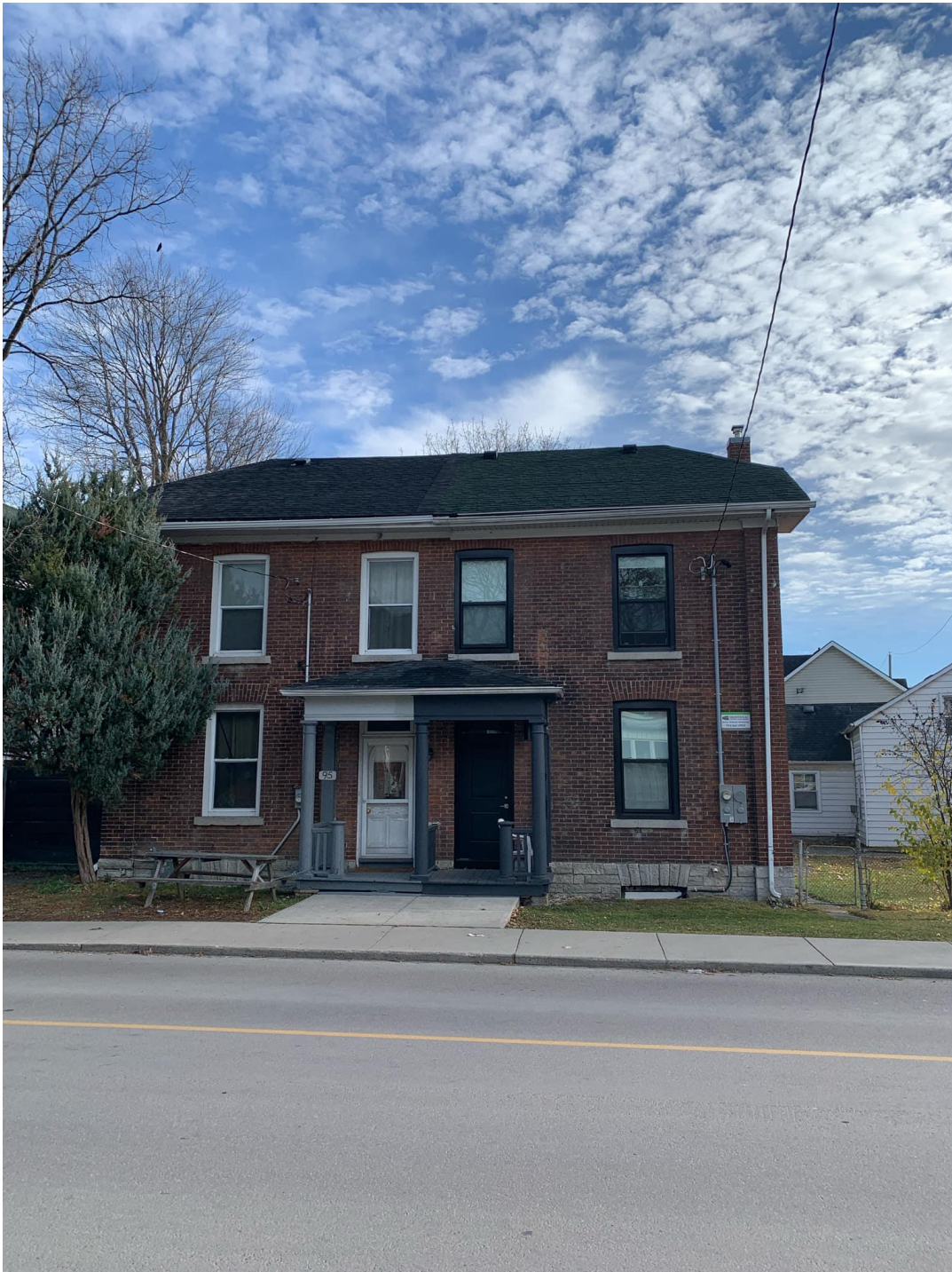
Figure 1: Front facing view of the of the subject property at 93 Division Street, and adjacent property at 95 Division Street, taken from the west side of Division Street (November 25, 2024).
