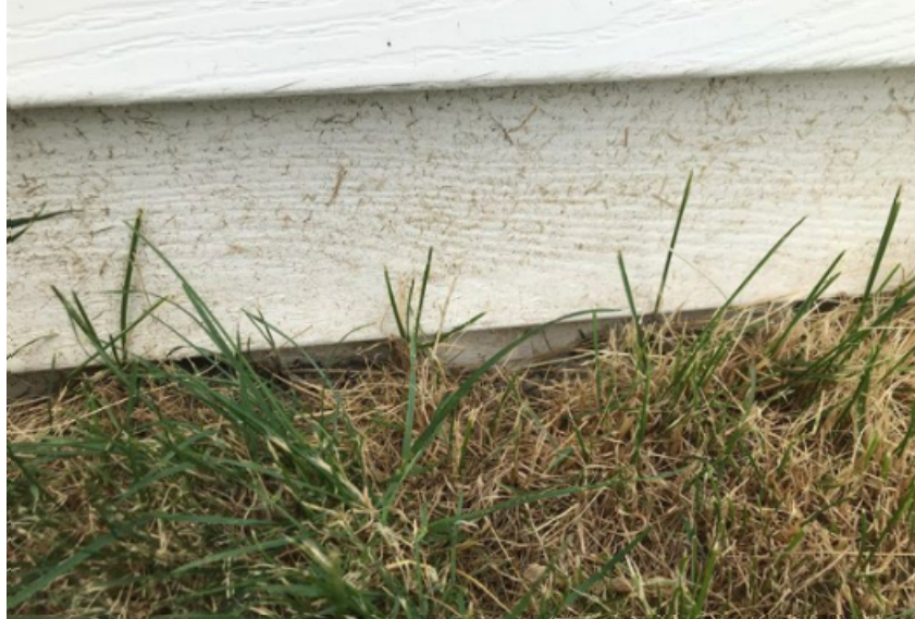
Figure 14: Vinyl siding extends under the sod on the east elevation, concealing foundation and demonstrating change in grade over time.
