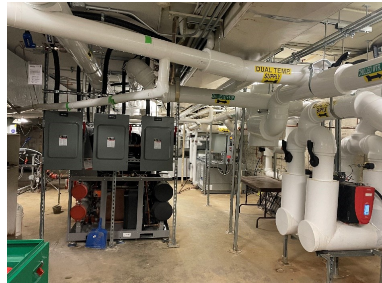
Figure 6. City Hall Mechanical Room
